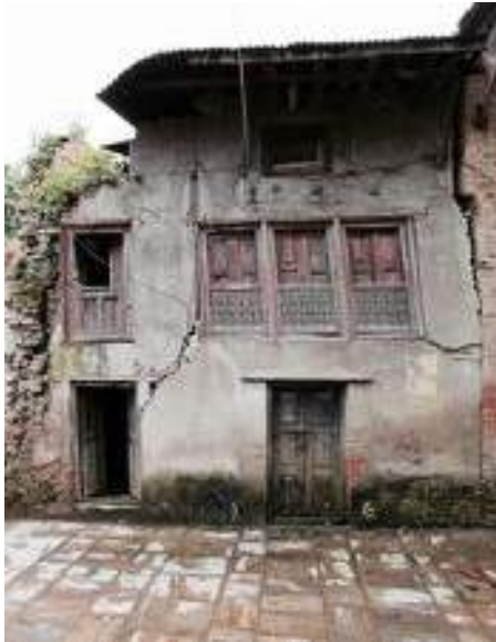
House still standing but the displacements are clearly visible, 2016
