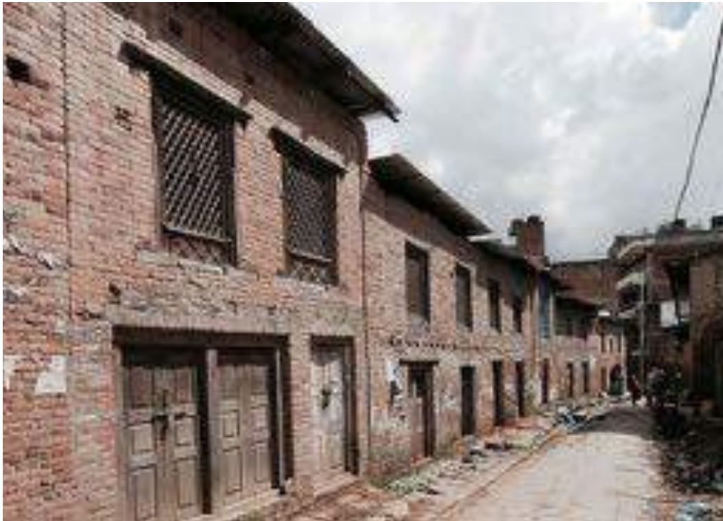
Entire row of Newari houses with removed upper floor in Khokana, 2016
