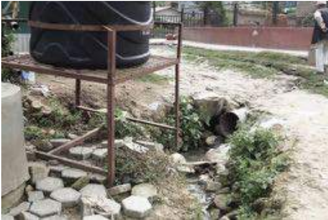
Part of the sewerage network in Bungamati, 2016
