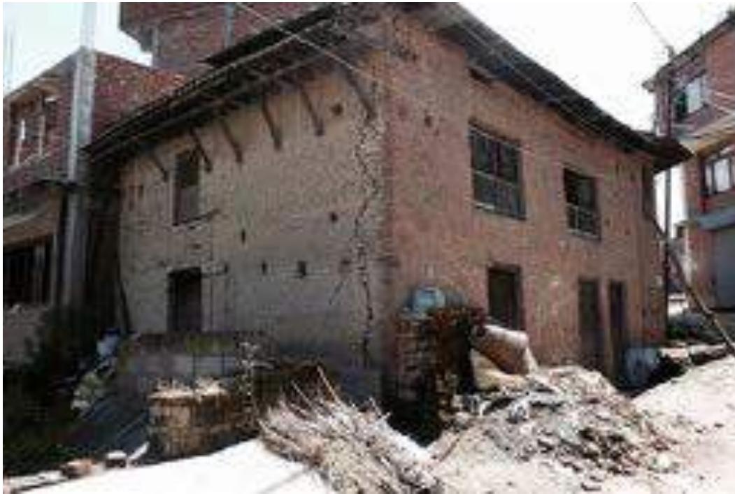
Cracks near the corner of a building in Bungamati, 2016
