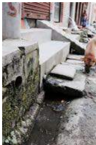
Lowered part of the road
