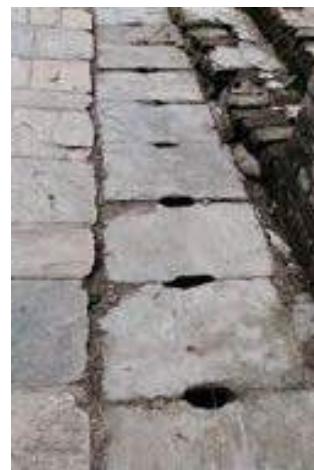
Fully covered sewage system
