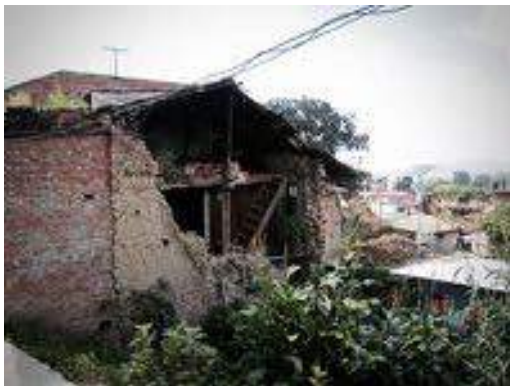
Damaged house in Bungamati, 2016
