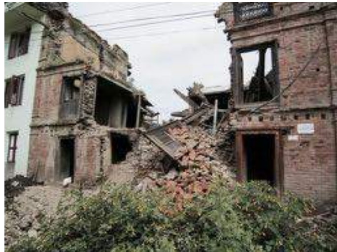
Collapsed house during the fieldwork in Bungamati, 2016
