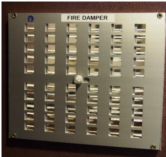
Figure 54 Fire damper of the engine room Source: own work
