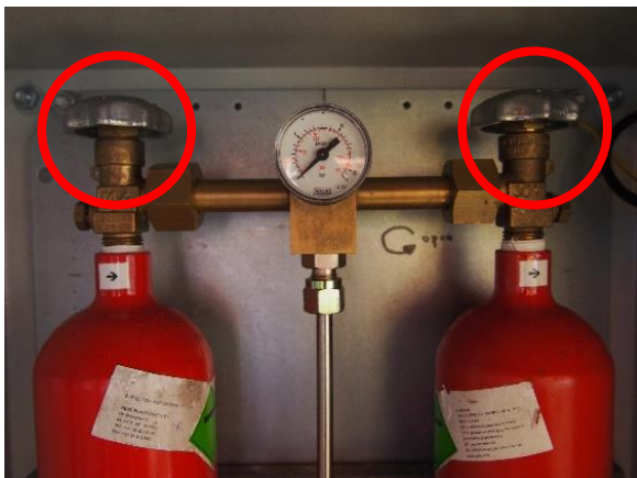
Figure 87 Opening of the pilot cylinder filling valves Source: own work
