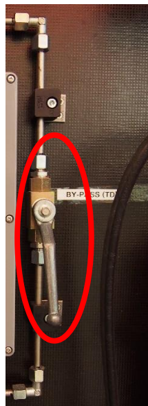
Figure 100 Bypass on the time delay unit Source: own work
