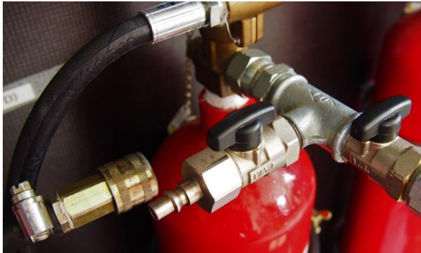
Figure 72 Compressor disconnected from the CO 2 filling piece
