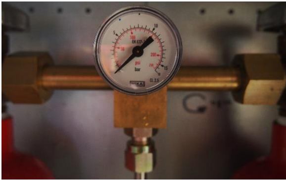
Figure 102 Pressure gauge on the pilot cylinders, indicating zero Source: own work
