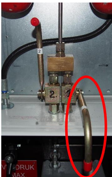
Figure 88 Activation of the main release valve, right lever Source: own work
