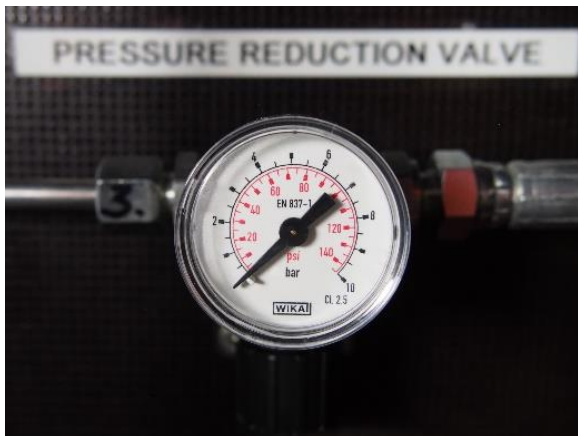
Figure 103 Pressure gauge on the pressure reduction valve, indicating zero Source: own work
