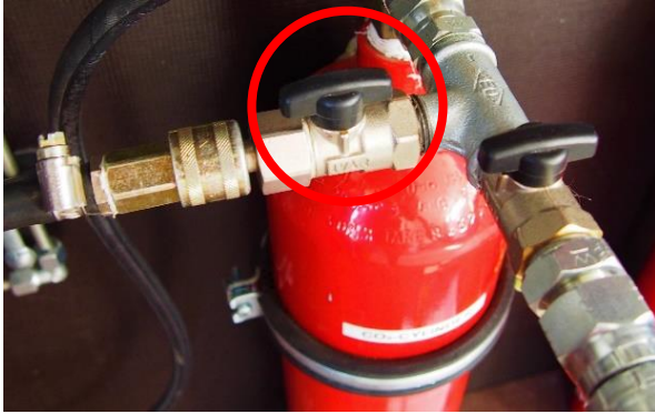
Figure 69 CO 2 filling piece, compressor connection open Source: own work
