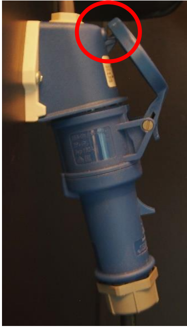
Figure 50 Power cable, plugged in Source: own work
