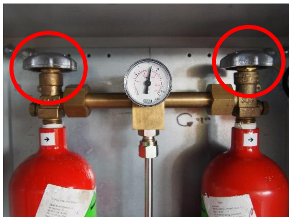
Figure 61 Closing of the pilot cylinder valves Source: own work
