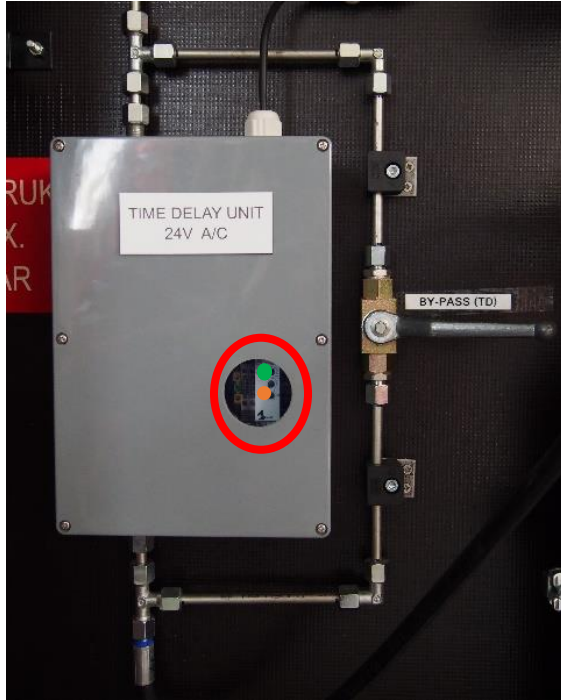
Figure 91 Time delay unit, activated Source: own work
