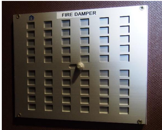
Figure 83 Fire damper from the engine room, close position Source: own work
