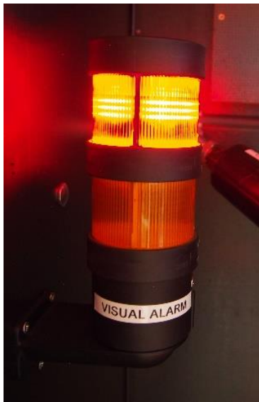
Figure 92 Visual alarm Source: own work
