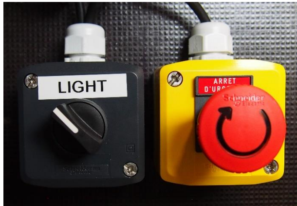
Figure 107 Light and emergency switch Source: own work
