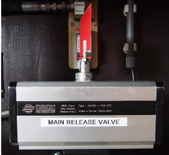
Figure 44 Main release valve, closed position Source: own work
