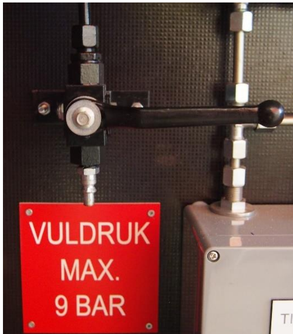
Figure 49 Pilot cylinders filling valve, closed position Source: own work
