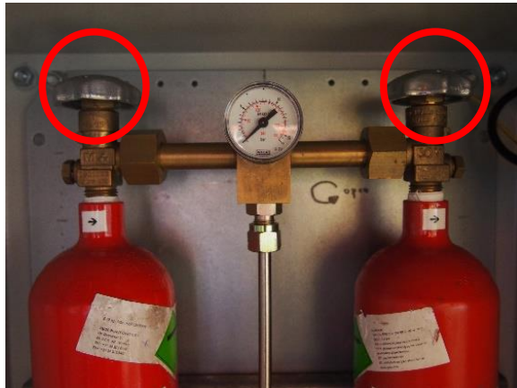
Figure 57 Opening of pilot cylinder valves Source: own work
