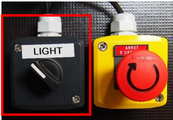
Figure 79 Light switch Source: own work
