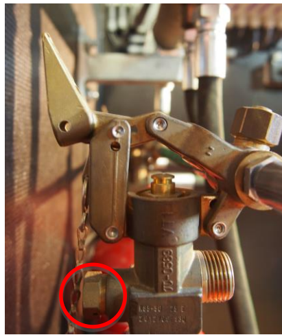
Figure 37 Bursting disc on CO 2 cylinder Source: own work
