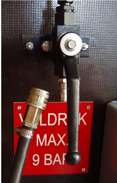
Figure 62 Disconnection from the pilot cylinder filling piece Source: own work
