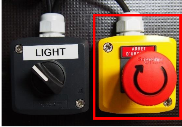
Figure 78 Emergency switch Source: own work
