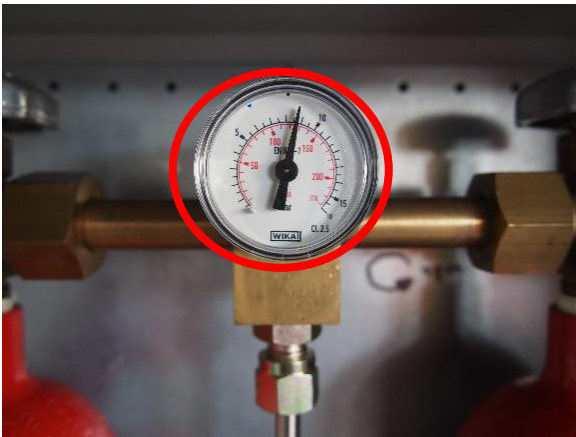
Figure 60 Pressure gauge on the pilot cylinders, indicating 9 bars Source: own work
