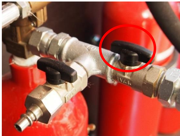
Figure 74 CO 2 filling piece, opened to the manifold side
