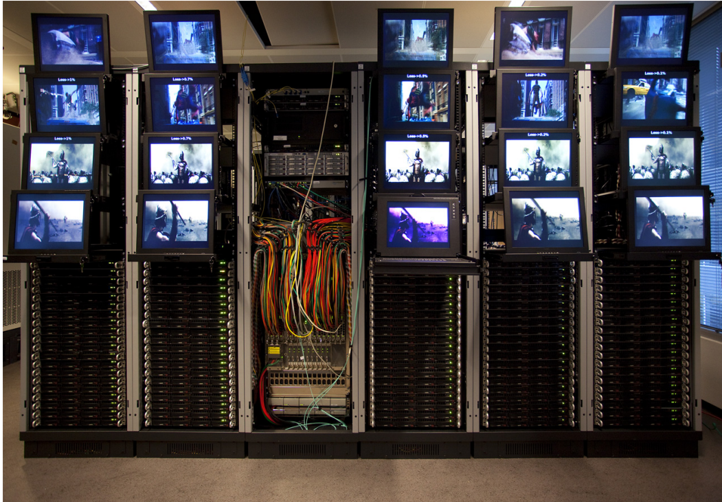
Figure 4.1: The Virtual Wall at IDLab Ghent. The Virtual Wall I has 206 nodes and the Virtual Wall II has 161 nodes at their disposal. Each node can be configured over SSH with the jFed tool.
