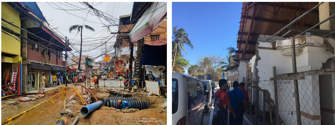
Figure 27 Photos of drainage repair and installation during rehabilitation (Arban, 2018) and of a partly demolished edifice near Bulabog Beach (own processing)
