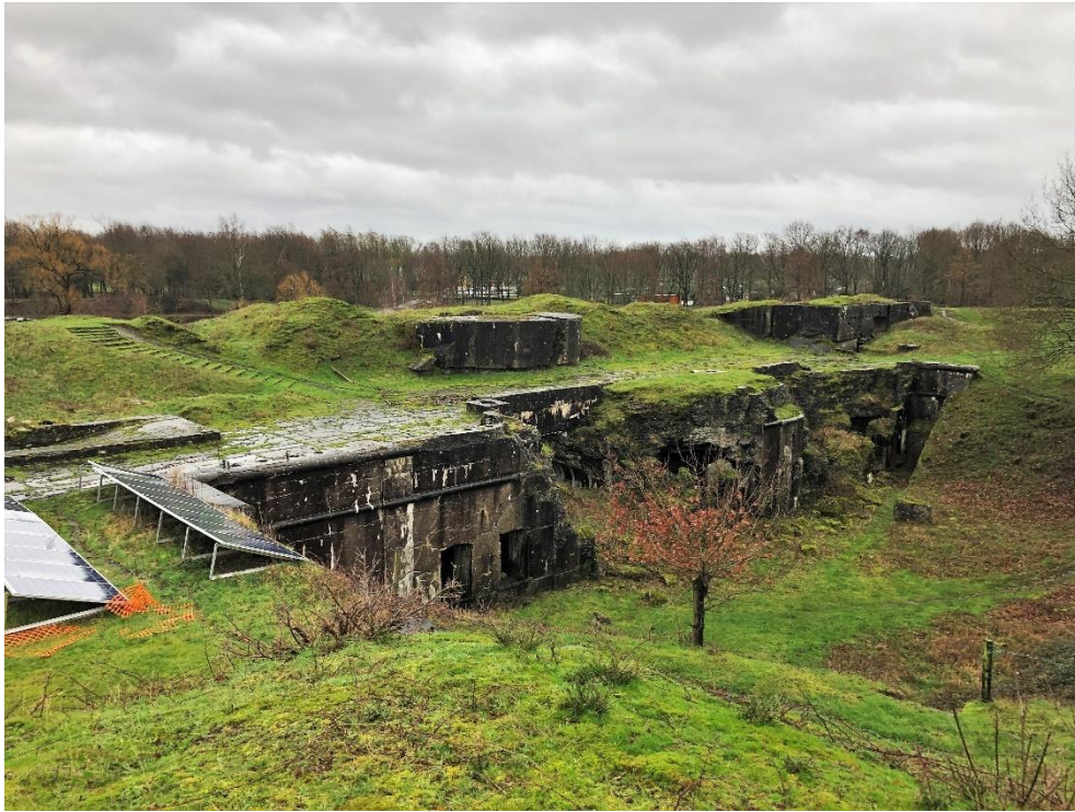
Figure 15 The existing situation of the Fortress of Kessel with a view towards the part of the principal front that is damaged during the First World War.
