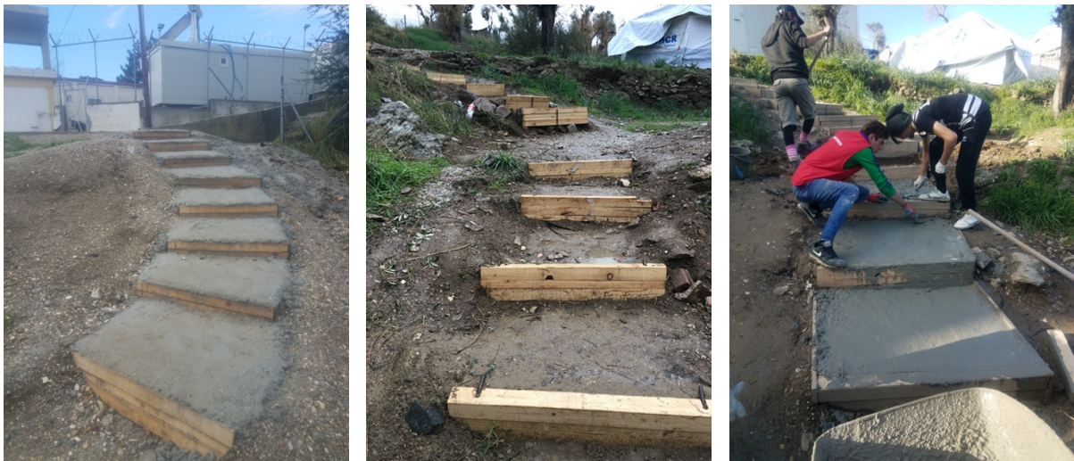
Figure 21: The stairs which were handcrafted in the second phase. However, in the end the army poured concrete on top of the stairs to make them more durable. (Source: ODD)
