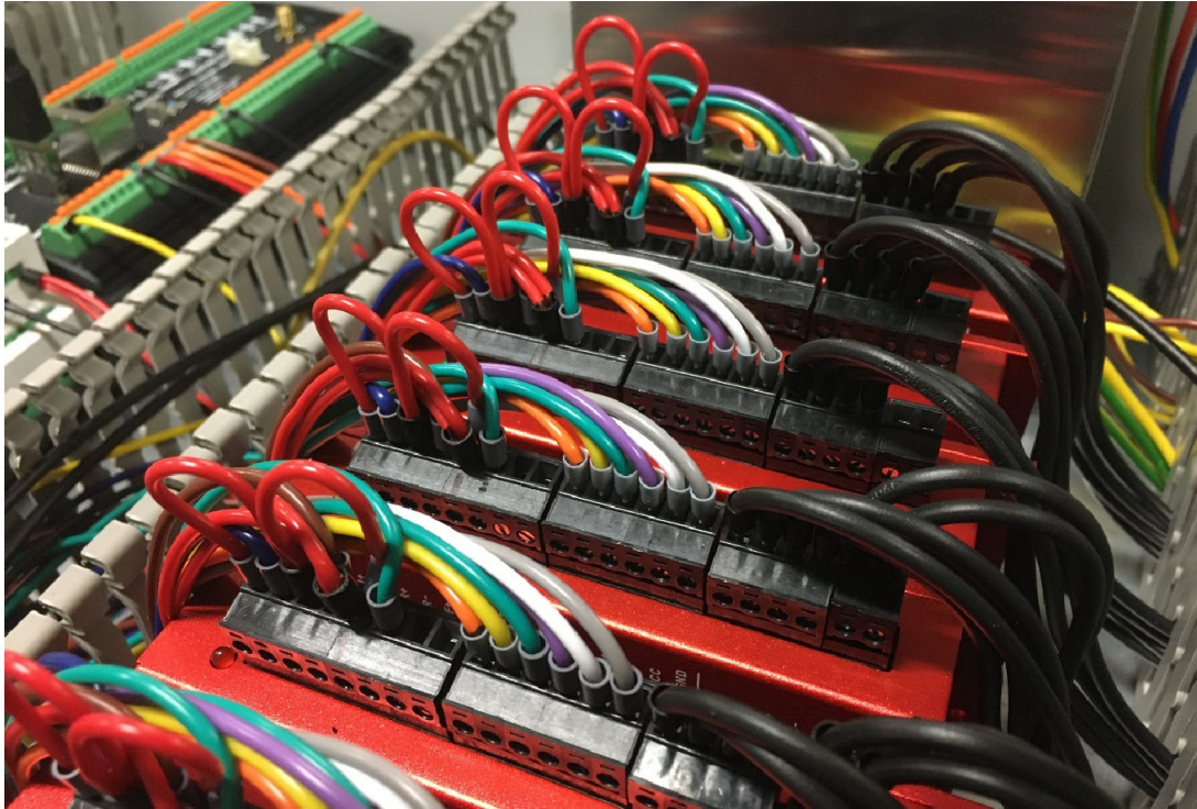
Figuur 78: Drivers in de schakelkast | Noot: copyright 2023 Bram Dupré
