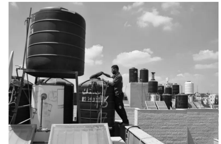
^ Illustration 37: Rooftop water tank.
