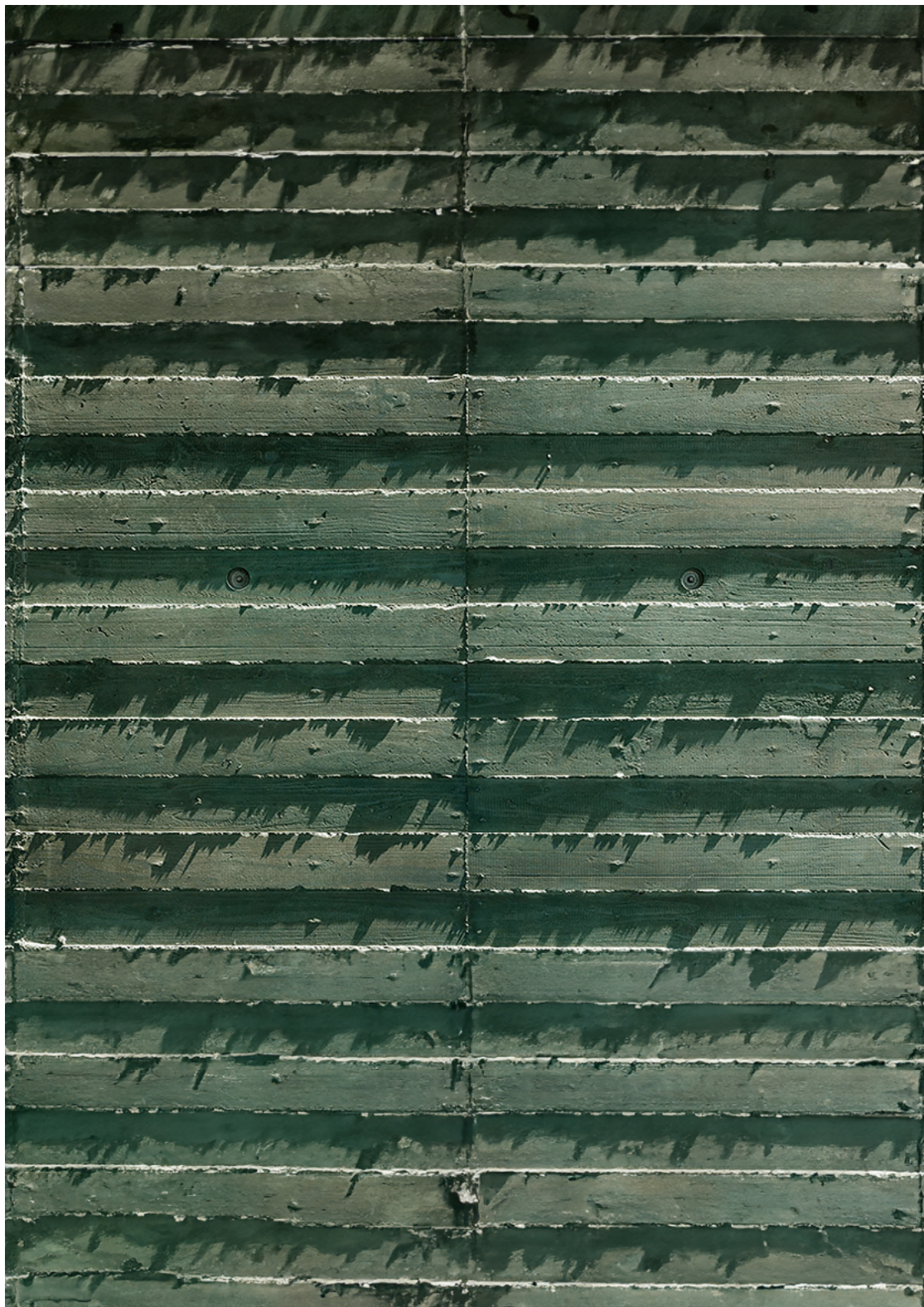
(fig.6.16) wooden board affected by salinity - corrosive impact resulting in uneven texture
