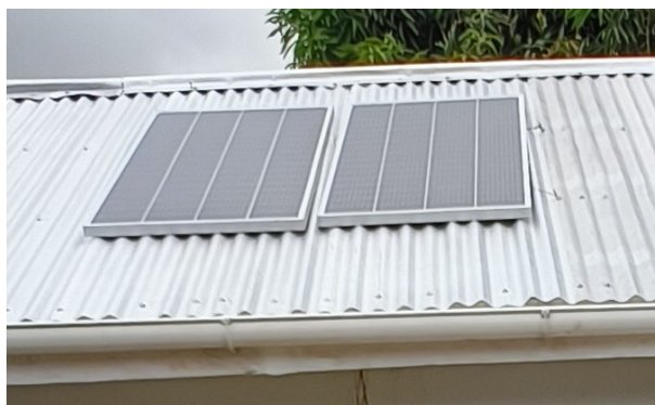
Figure 5.10: Solar panels mounted on roof
