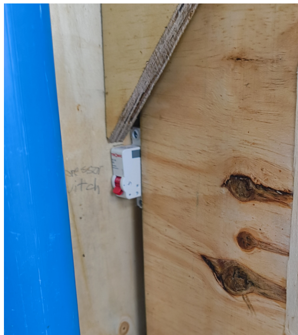
Figure 5.12: Circuit breaker used as main switch
