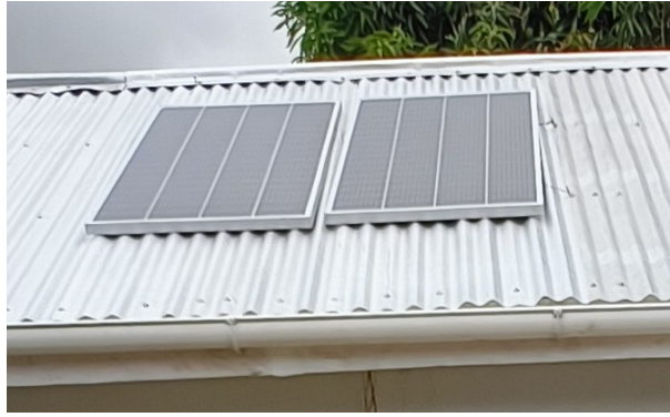
Figure 5.2: Selected solar panels
