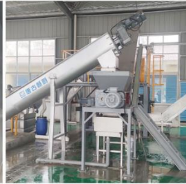
Conveying & Shredding System
