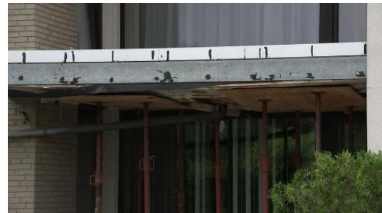
Figure 1: Decay –deteriorated balcony https://www.vrt.be/vrtnws/nl/2022/05/10/appartementen-met-houtrot-in-sint-truiden-worden-best-afgebroken/
