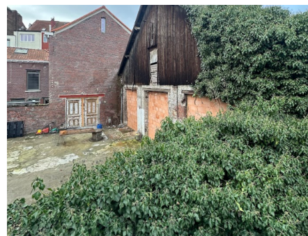
fig [5.39] Warehouse shed with exterior wall with overgrown plants
