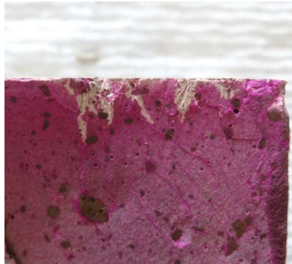
Figure 68: Carbonation around very fine shrinkage cracks in cement paste; 12 weeks of exposure
