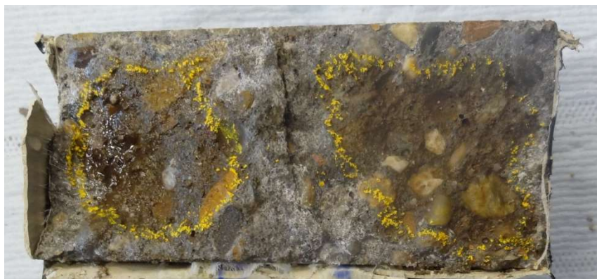
Figure 55: Classification of the chloride penetration profiles in four classes: A) equidistant penetration from the surface B) local penetration around crack C) chloride penetration up to the opposite coated side D) chloride penetration up to the opposite coated side accompanied by accumulation of chlorides at the coated side; The chloride penetration is from the top of the picture
