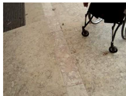
Figure 48 Step at the Exit
