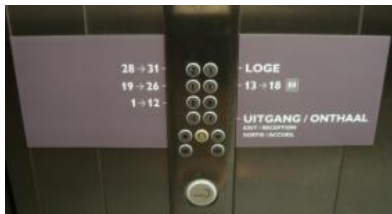
Figure 200 Elevator of Museum M
