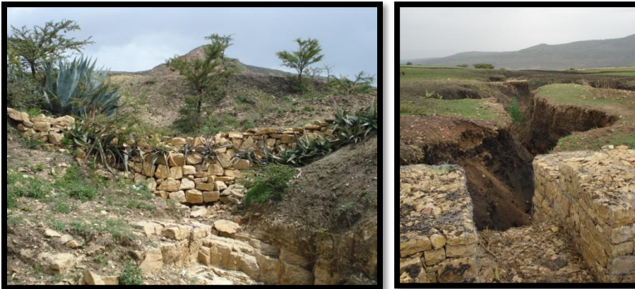
Figure 2.10 Check dam (left) and gabion (right) for gully erosion control in the Mayleba catchment, (August, 2011)
