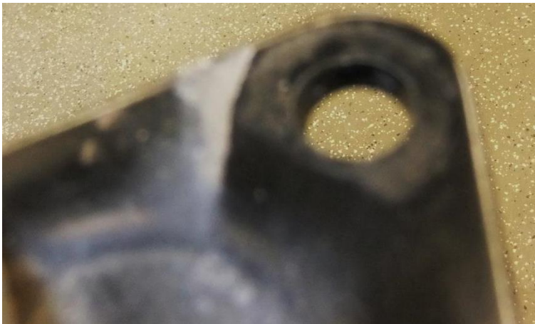
Appendix Figure B 21: Roll restrictor bracket coating damaged by movement between the component and the gearbox, reverse side of the figure above
