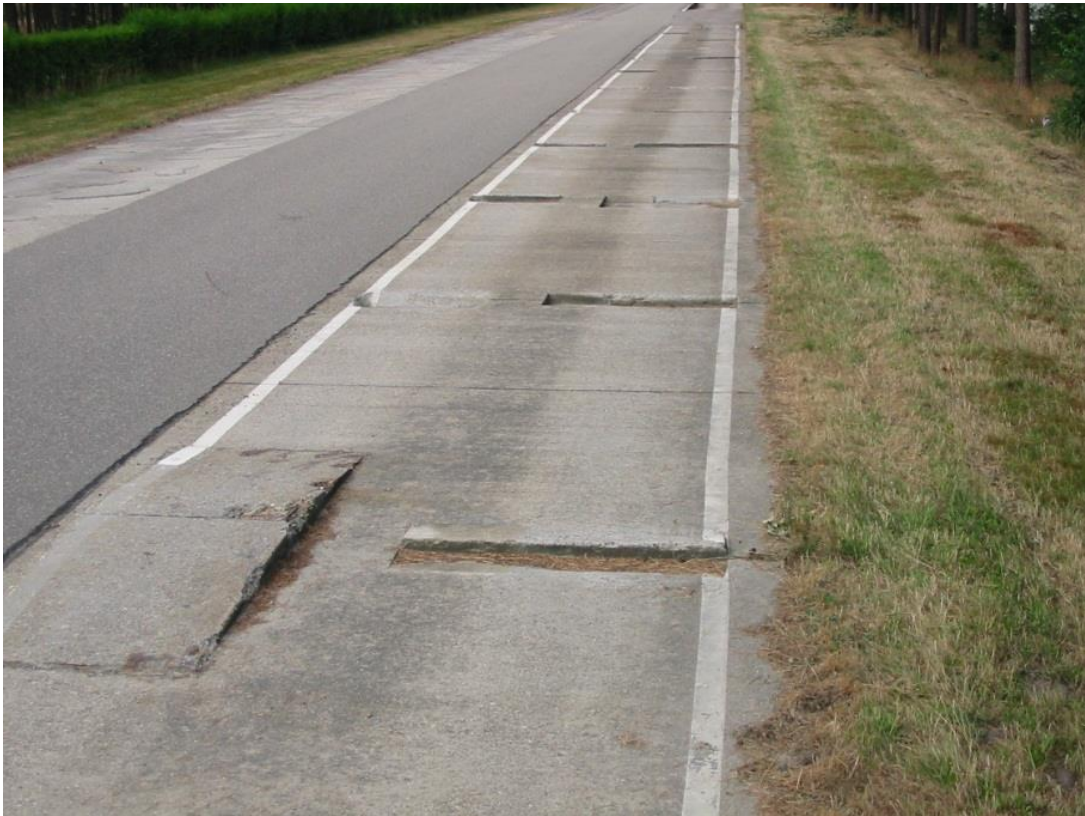
Appendix Figure B 4: Chuckholes lane
