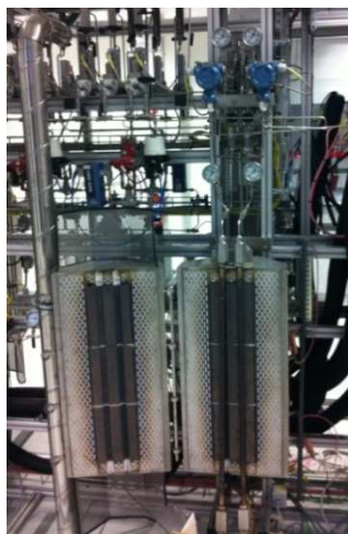
Figure 2-1: HTK-1: reactor grouped in one furnace
