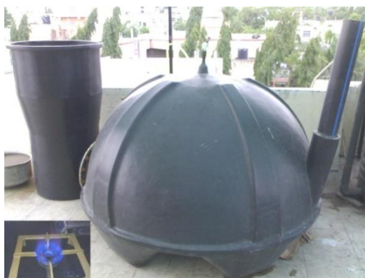
Figuur 6: VIVAM biogasinstallatie [13]
