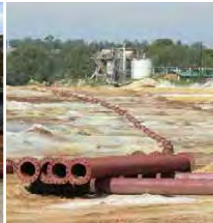
sludge transport in pipes
