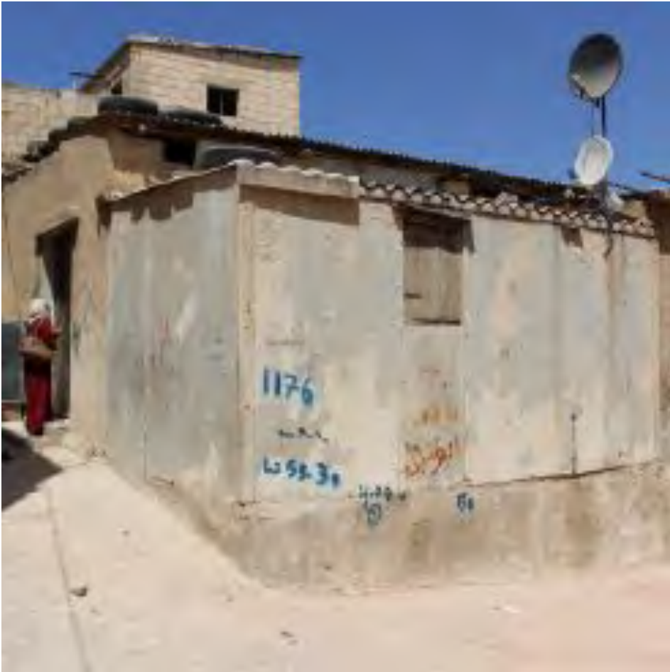
An example of one of the remaining asbestos units.
