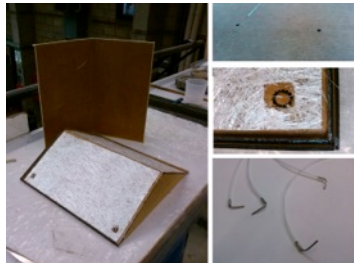
Place and impregnate 300 gr/m 2 glass-fibre mat; place and redirect the PVC air-tubes; bend steel tubes at endpoints of some PVC air tubes; pitch roof
