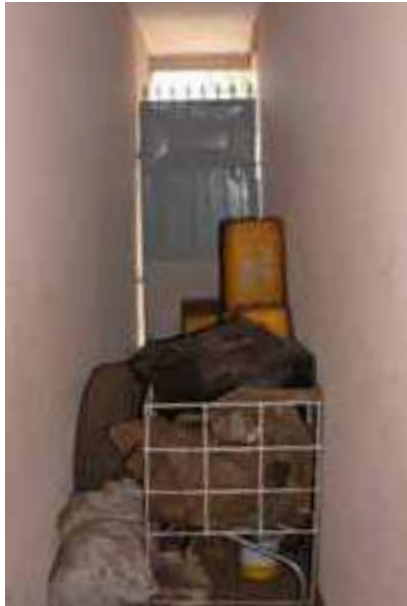
The side entrance is blocked by personal belongings of the residents.
