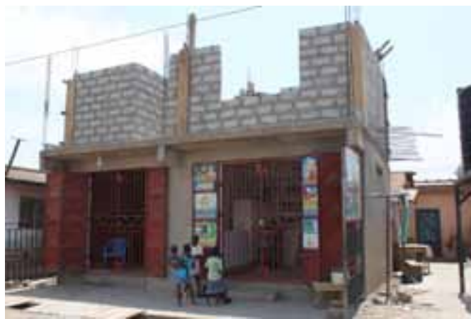
Two-storey building in construction. The ground floor is reserved for commercial units.
