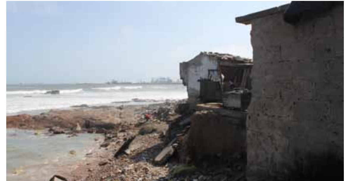
Sea erosion is threatening the houses in Awudung.
