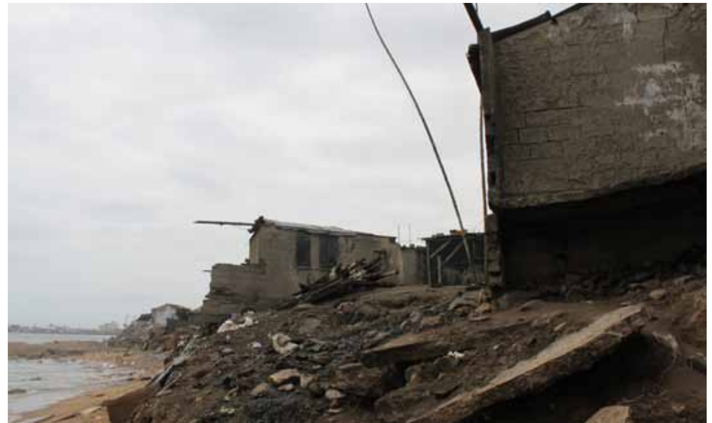
The current situation in Awudung: the erosion causes severe damage.
