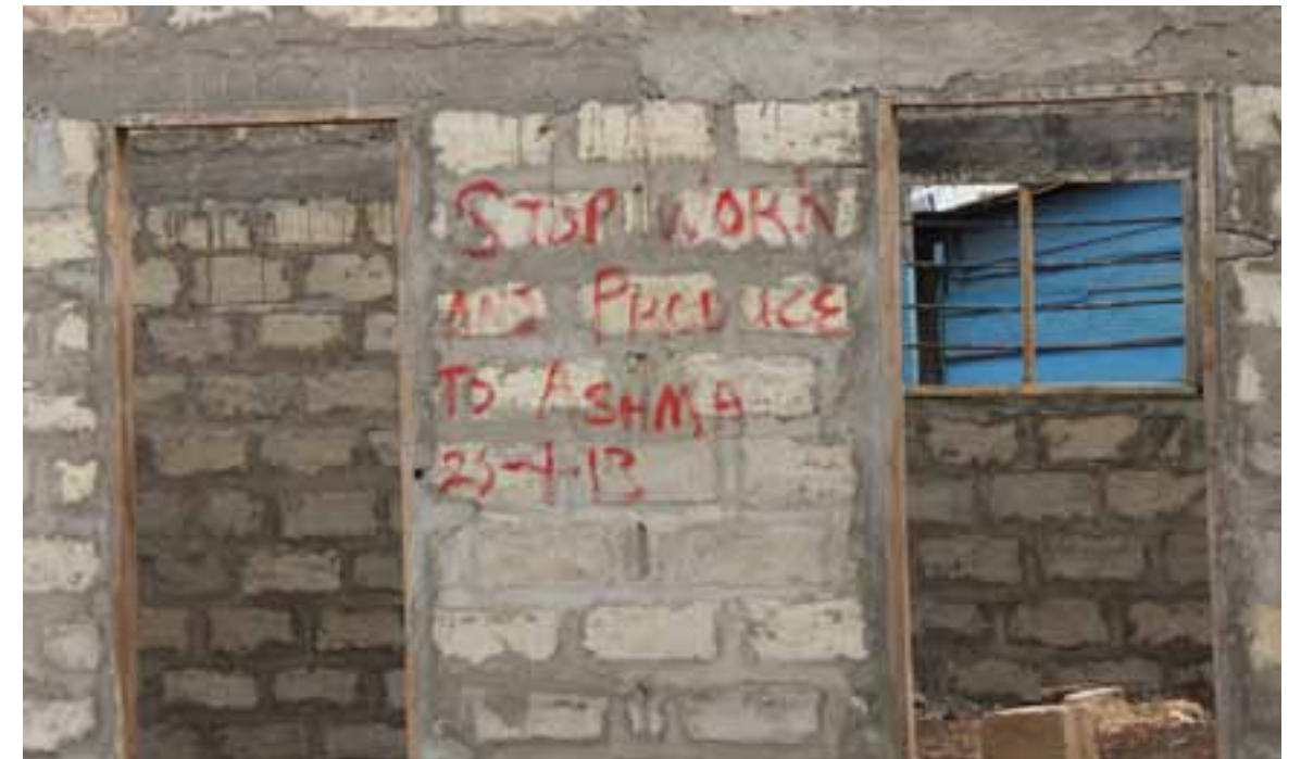
ASHMA commanding residents who started construction to produce a permit for the property.
