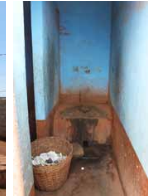
Public toilet owned by TMA and managed by a committee of residents.
