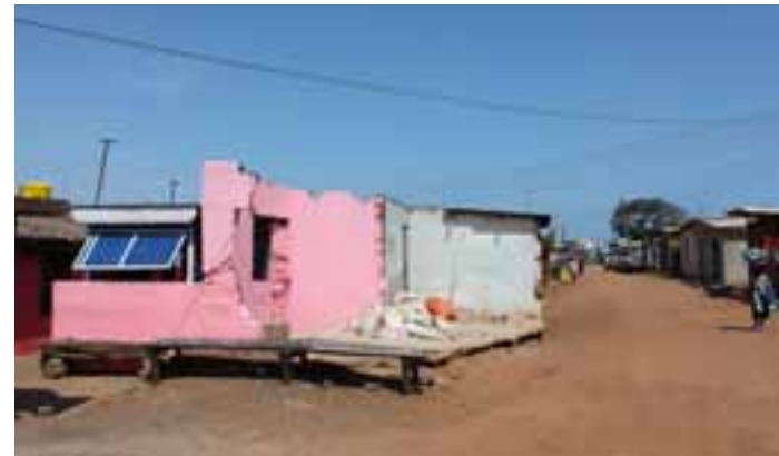
A resident living in Manhean lost a part of his house since it was standing on the demarcation of a road.
