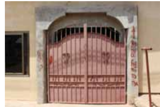
Marking by TDC to warn a member she has to produce a building permit (they thought she was constructing a second storey).
