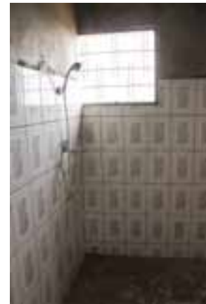
Shower under construction in a three-storey house in the low-cost area. (D/17)
